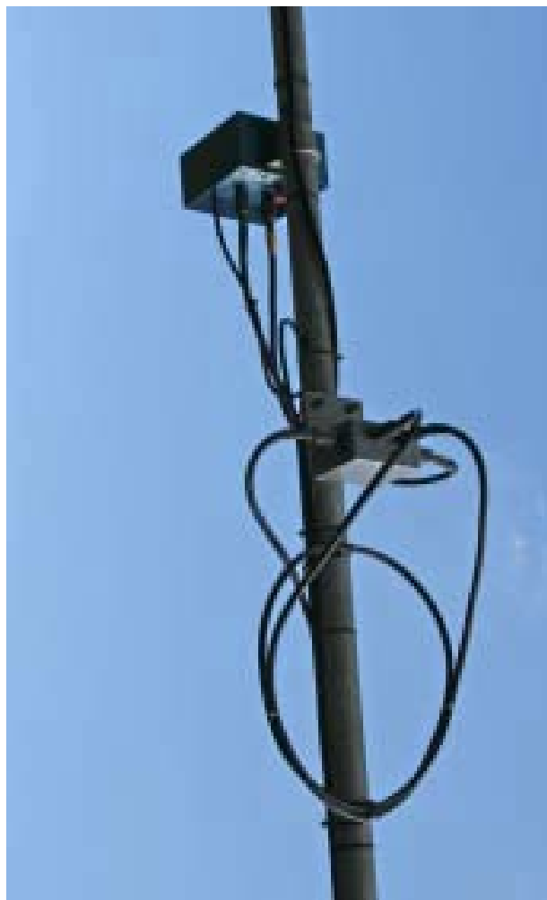
The Stackmatch and Phase Shifter mounted on the tower.
