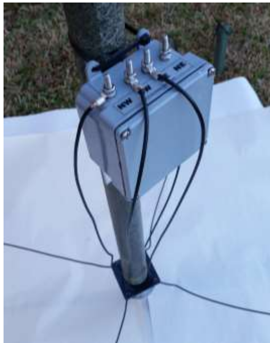
View of the bottom section of mast and relay box installed with the two loops connected.
