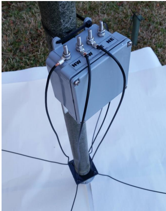
View of the bottom section of mast and relay box installed with the two loops connected.
