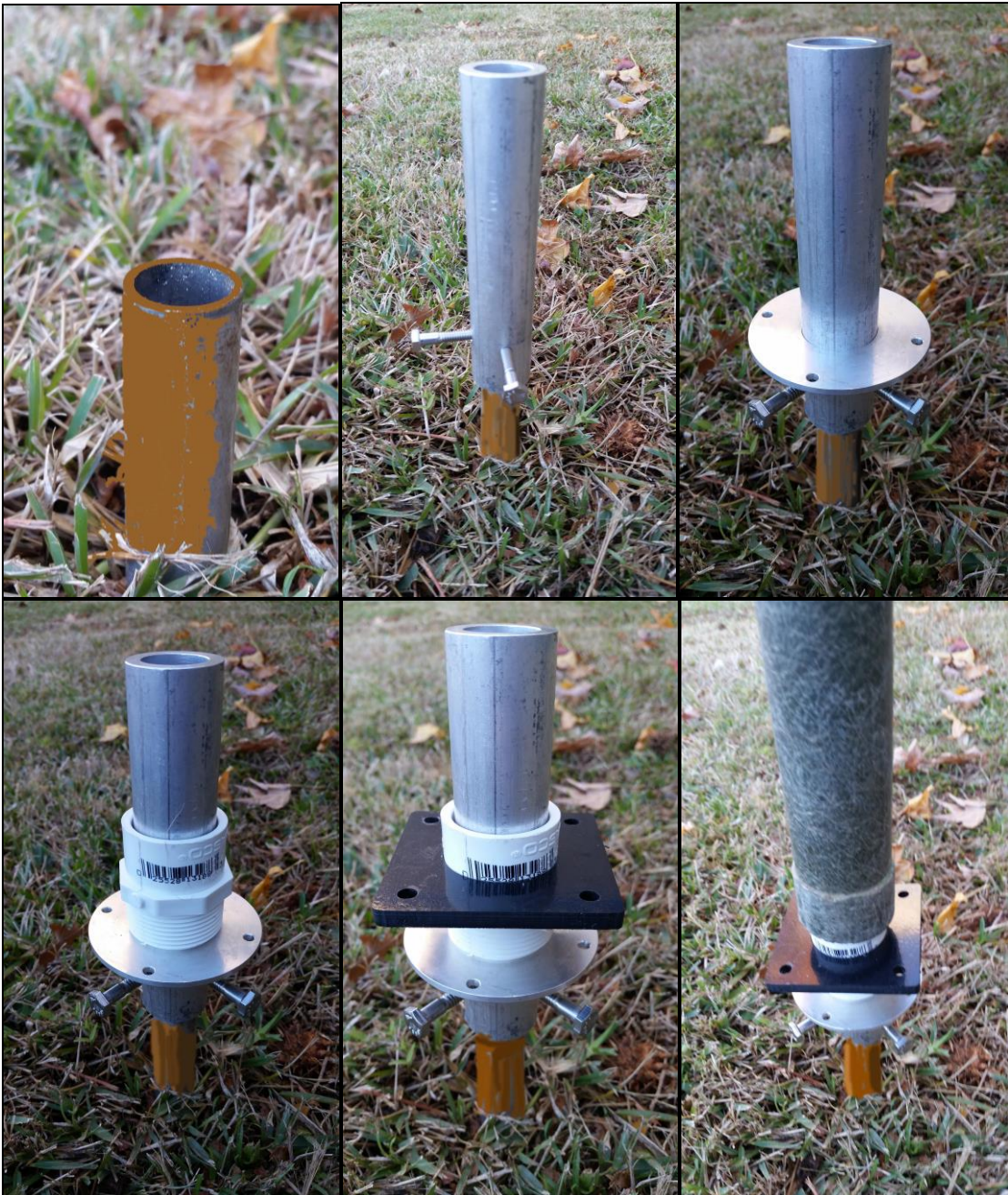
Sequence of base assembly, from the grounding rod to the first mast pipe section
